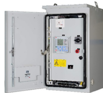
LV control cabinet
